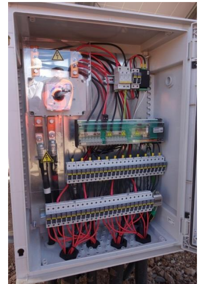
Visual inspection of combiner box
